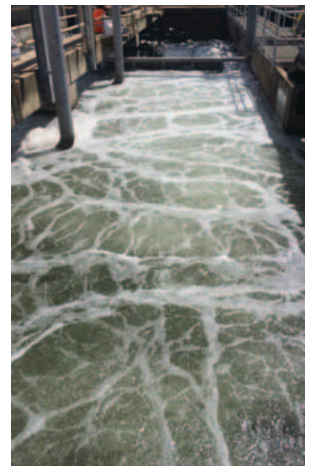
Aerostrip® fine bubble diffusers in operation at Rockhampton STP.
