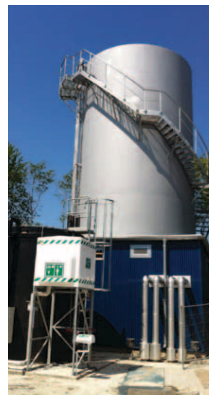
CNP plant installed in Weiden, Germany.
