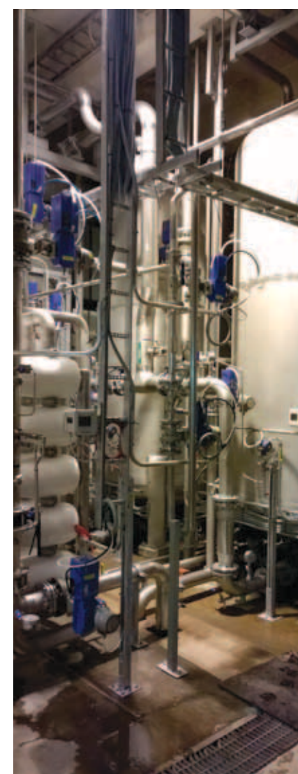
Flootech demineralized water treatment system at Stora Enso Varkaus Power Plant.
